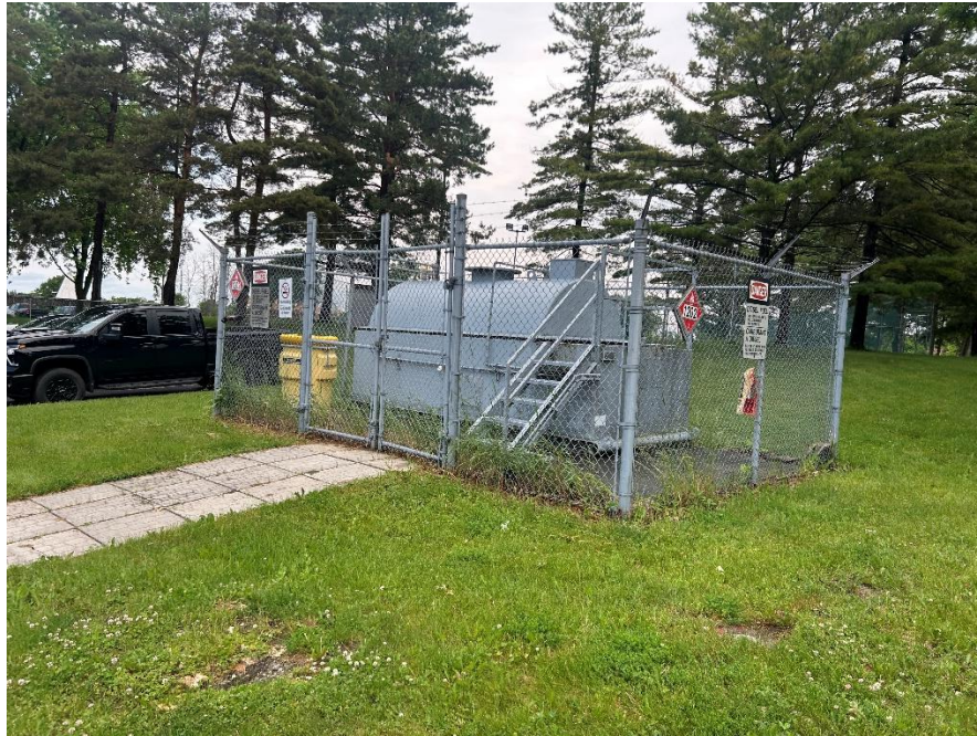
Photo 9 Diesel AST east of Site Building A, June 10, 2025.
