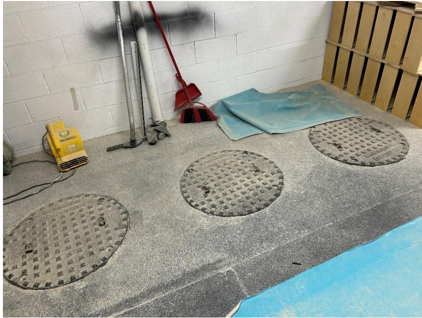
Photo 5 Oil/water separator within the vehicle servicing garage in Site Building A, June 10, 2025.
