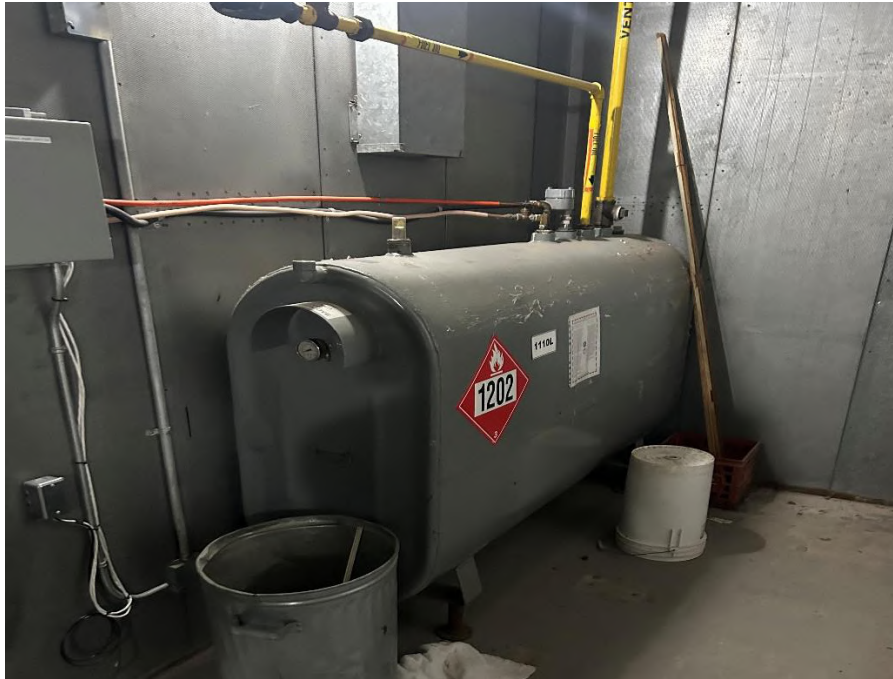
Photo 7 Day tank diesel AST in the vicinity of the emergency generator in Site Building A, June 10, 2025.
